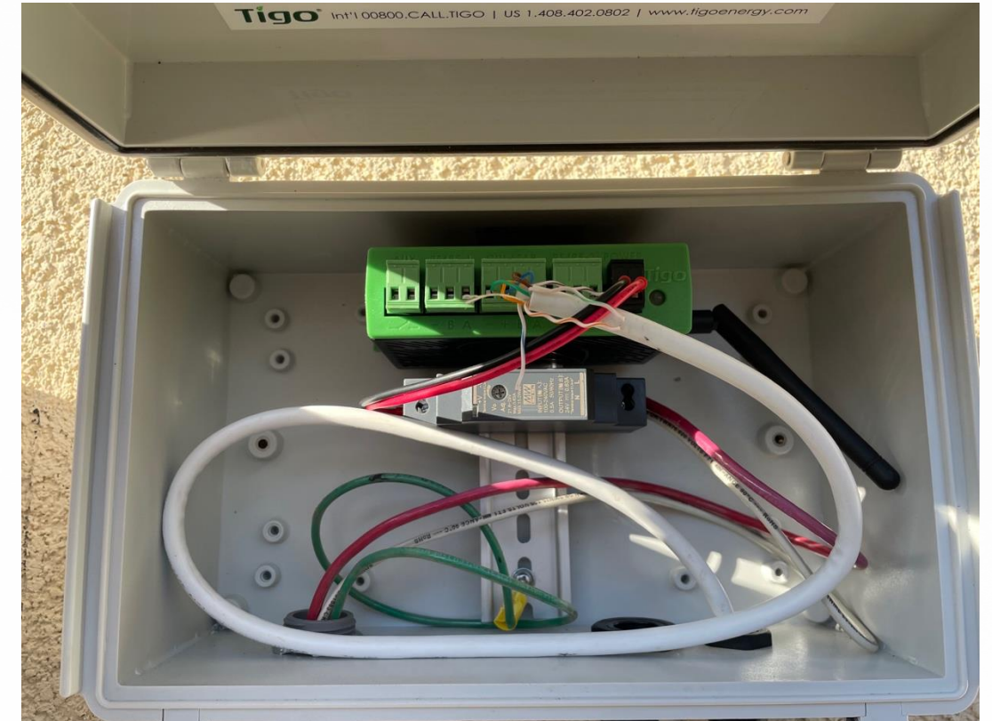
Properly installed CCA in IP68 Enclosure
