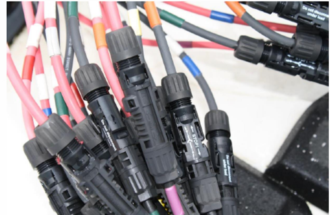
Cap screws not tightened enough
