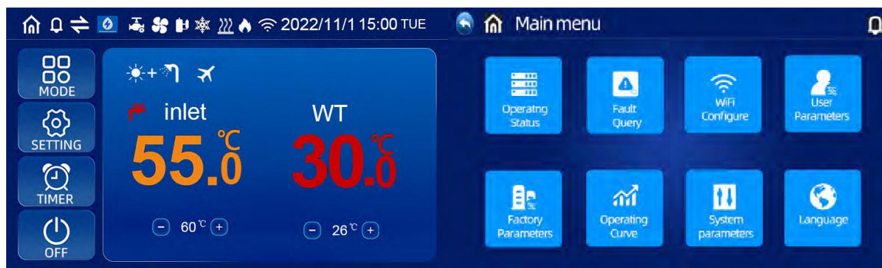
Touchscreen Controller – Home Screen
